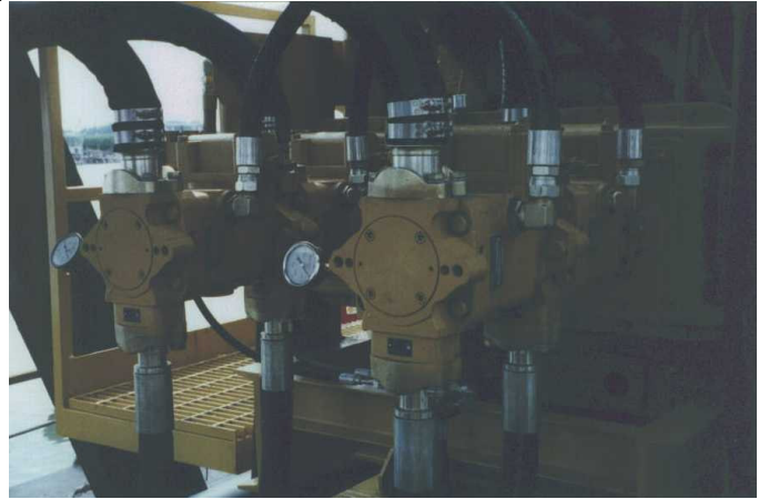
Hydraulic Drive Pumps
